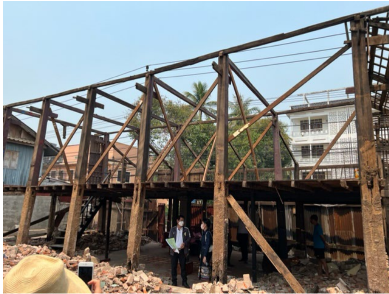
Reconstruction of a Lao traditional timber house, showing remaining salvageable parts and the advanced decay of the foundations of wooden pillars
